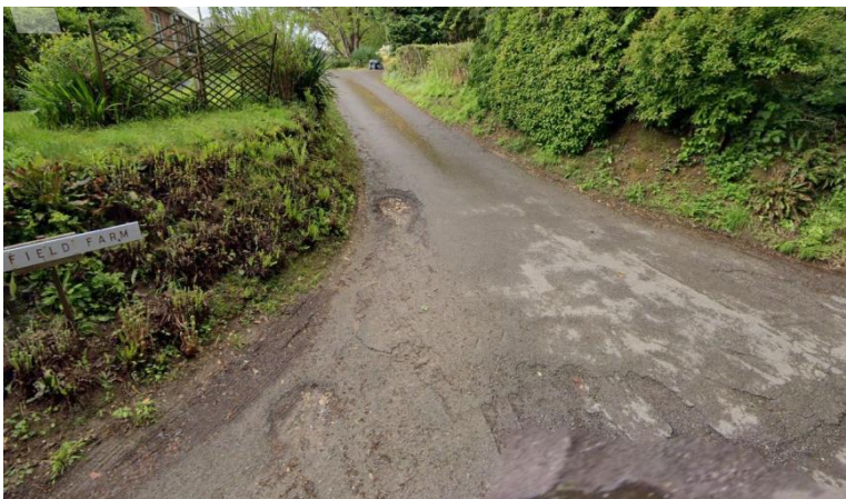
The narrow existing farm track slopes steeply at its junction with Puddletown
